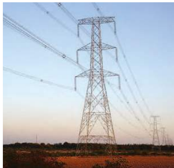
765 kV DC Kudgi Transmission Line project
