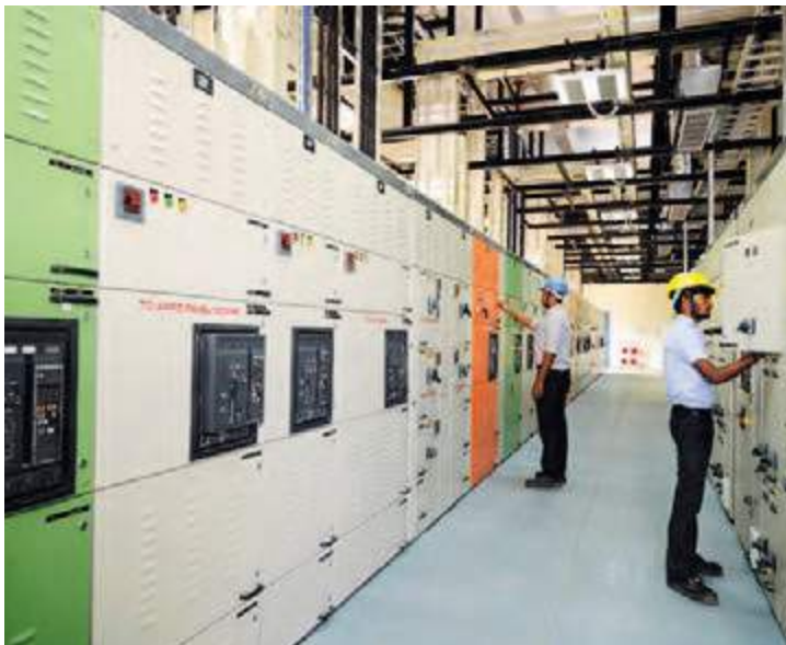
Switchboard installation at a national infrastructure site
