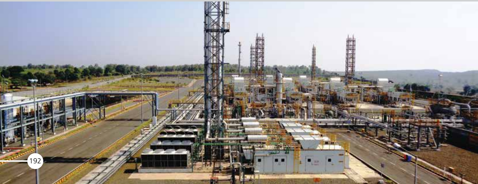
Group Gathering Station-11 for RIL's Coal Bed Methane Field Development Project at Shahdol, Madhya Pradesh, India
