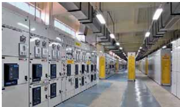
Switchboard installation at a power plant. L&T provides power distribution and control solutions – including LV and MV switchboards – across the value chain, from point of generation to end-user.
