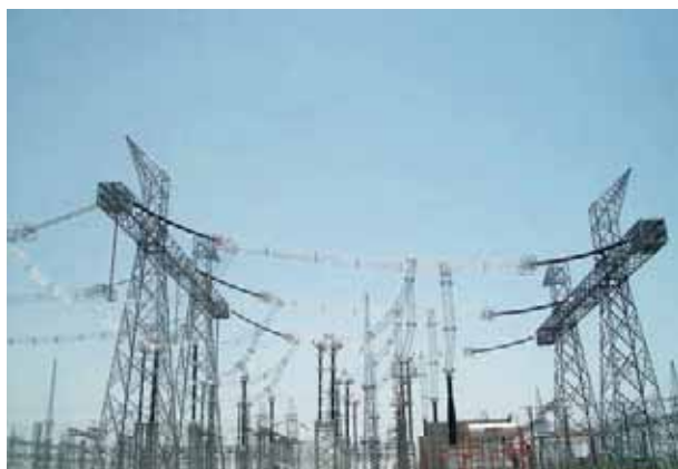
India's first 1200 kV substation at Bina in Madhya Pradesh built by L&T.
