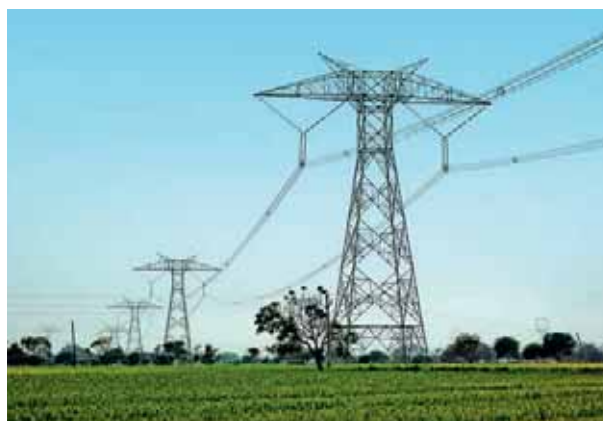
800 kV transmission lines between Nidhura and Agra.
