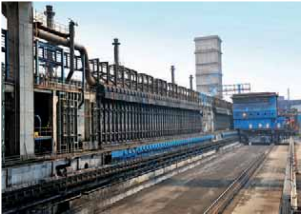
Coke oven battery executed by L&T for one of India's major steel plants.
