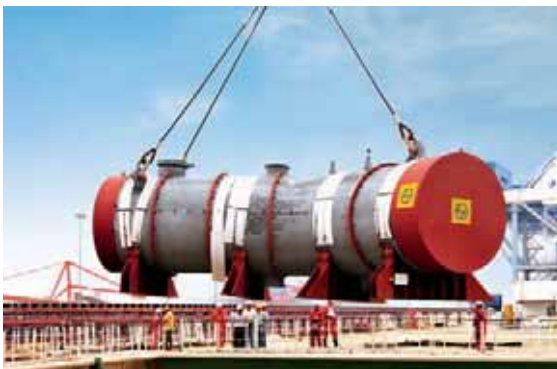
Coal gasifier being exported to China
