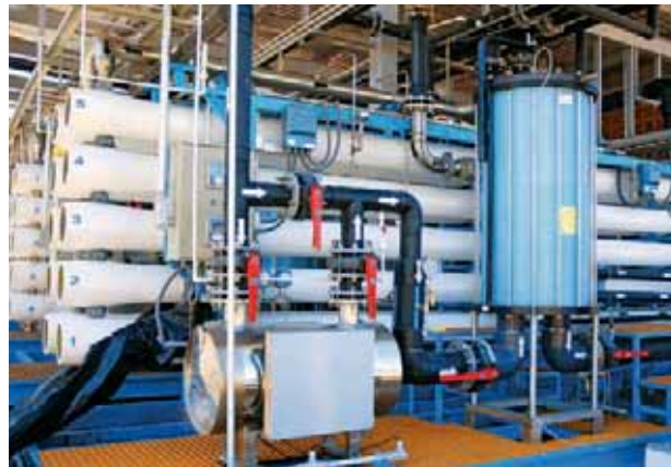
Reverse osmosis technology in operation at desalination projects.
