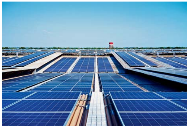
World's largest single rooftop (7.5 MWp) solar power plant in Punjab
