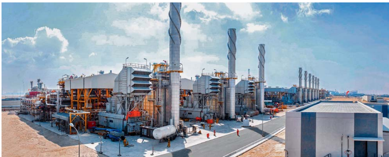
Upgrade project executed on an EPC basis for export gas compression facilities in Qatar
