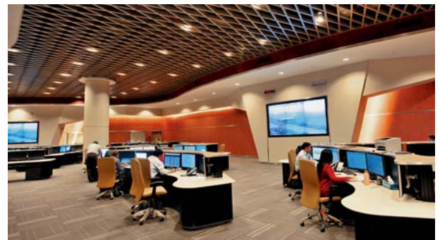
Mumbai International Airport Network Operations Centre - powered by L&T's control and automation systems and expertise
