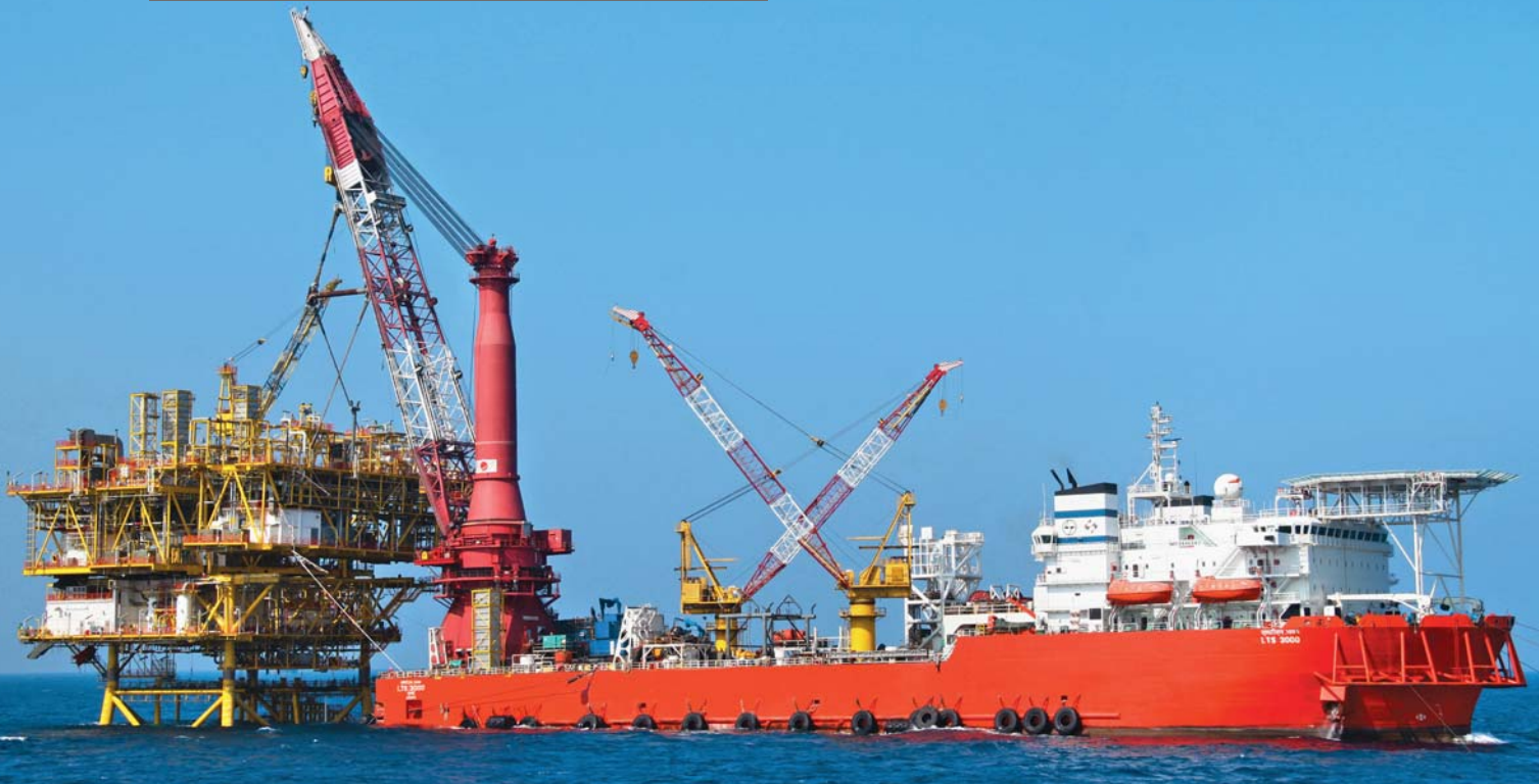
3000-tonne captive installation and pipelay vessel installs a wellhead platform off the coast of Myanmar
