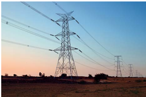
765 kV DC transmission lines at Kudgi, Karnataka
