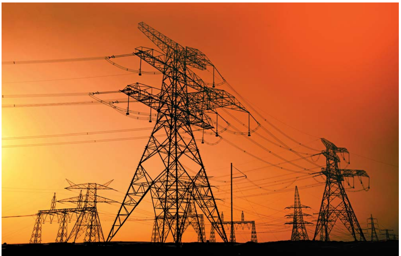
400 kV Bab Asab - Habshan Transmission Line in Abu Dhabi. L&T is one of the industry leaders in turnkey construction of power transmission and distribution systems in the Middle East.
