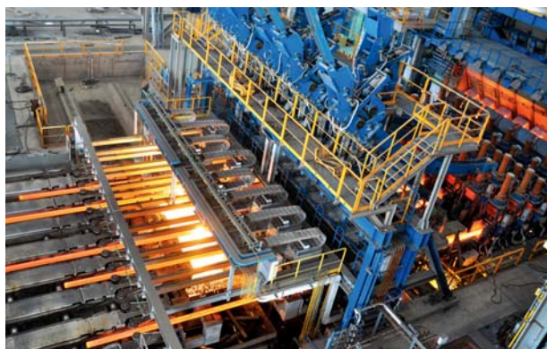
Steel Melt Shop for a steel major in Oman
