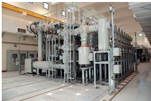
Electrical installations at a gas-based industrial substation in Doha
