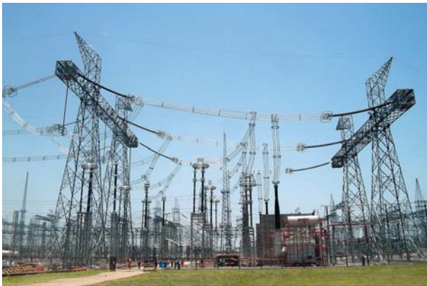
India's first 1200 kV substation at Bina, Madhya Pradesh. L&T offers complete solutions in high-voltage substations and power transmission lines.
