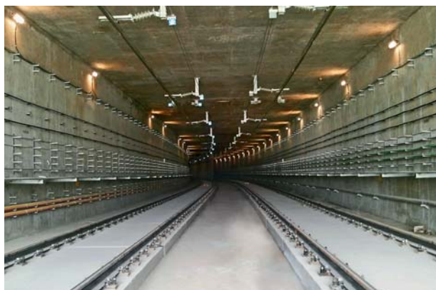
Rigid Overhead Contact System of Delhi Metro Rail Corporation
