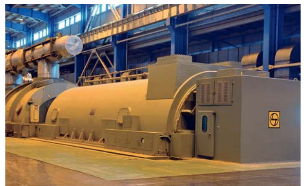
Enclosed turbine at a supercritical power project
