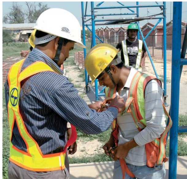
Safety is accorded top priority. Safety practices are rigorously implemented at all project sites around the country. L&T has also set up a unique Safety Innovation School at Hazira.
