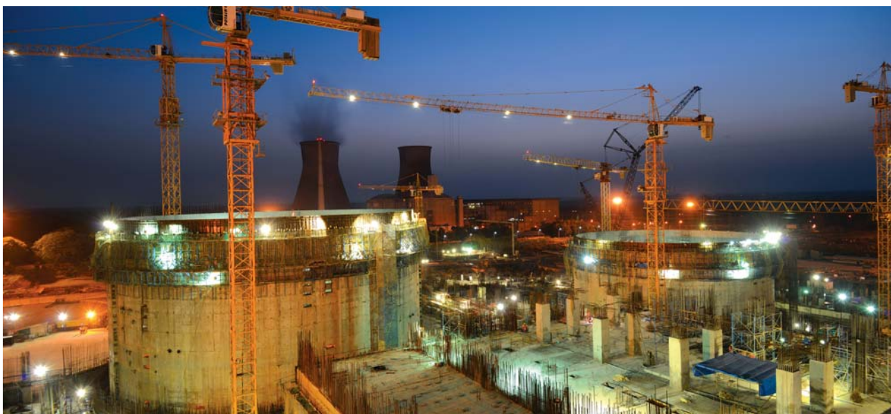
Construction of a critical structure in progress at Kakrapar Nuclear Power Project in Gujarat
