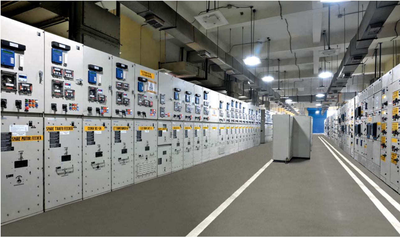
Switchboard installation at a power plant. L&T provides power distribution and control solutions across the value chain, from generation to end-user
