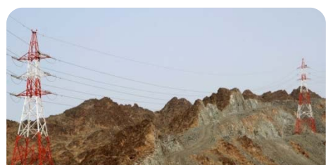
Transmission Lines, Al Majlis, Oman
