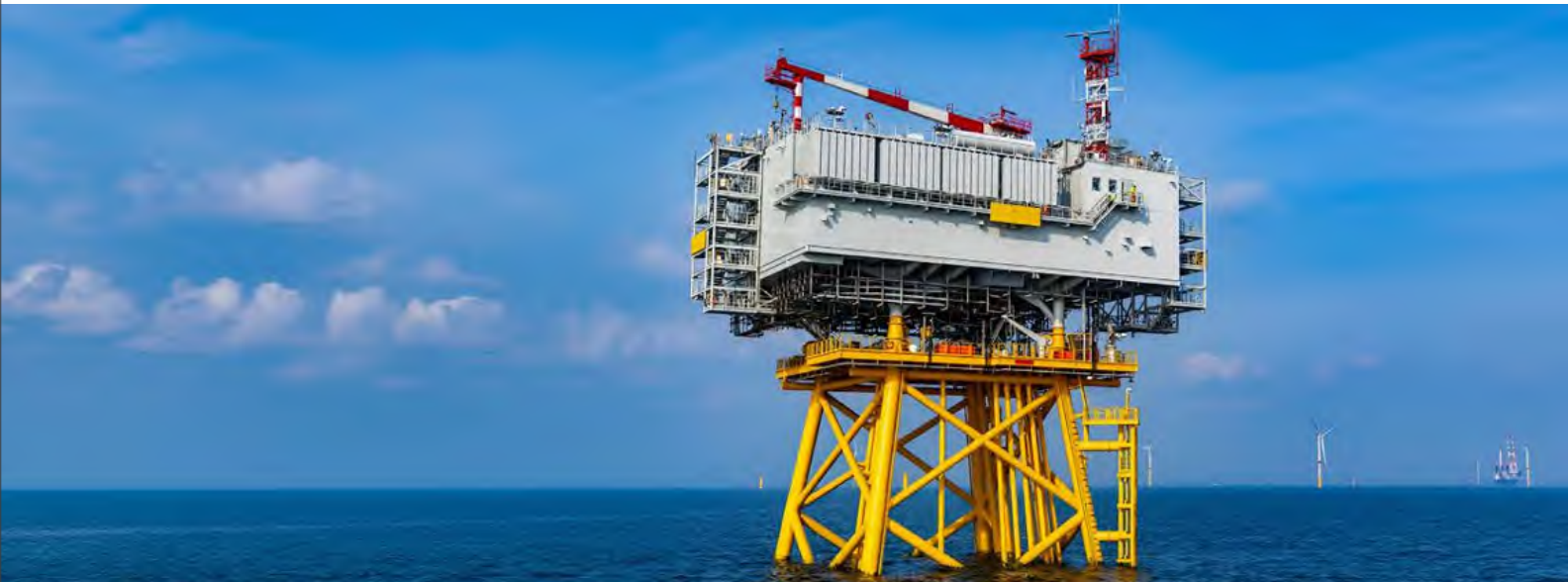
HVDC Offshore Substation
