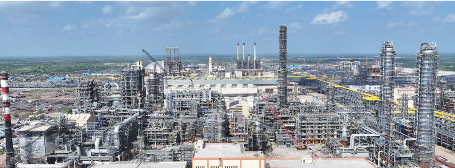
Petrochemical Fluidised Catalytic Cracking Unit & Propylene Recovery Unit for HPCL Rajasthan Refinery Limited (HRRL), Barmer, Rajasthan
