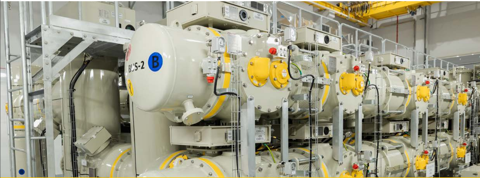
132 kV ESKAN YALAYIS Substation, UAE
