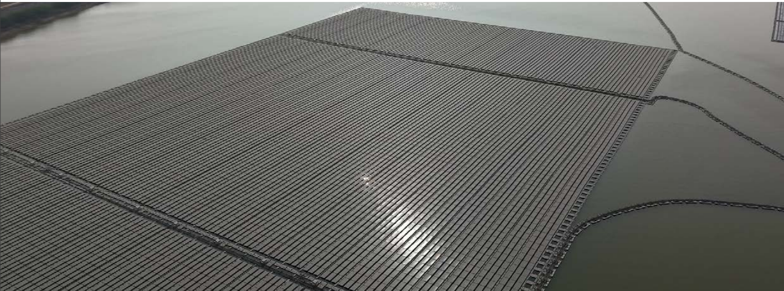
56 MW Floating PV Project, Ramagundam, Telangana
