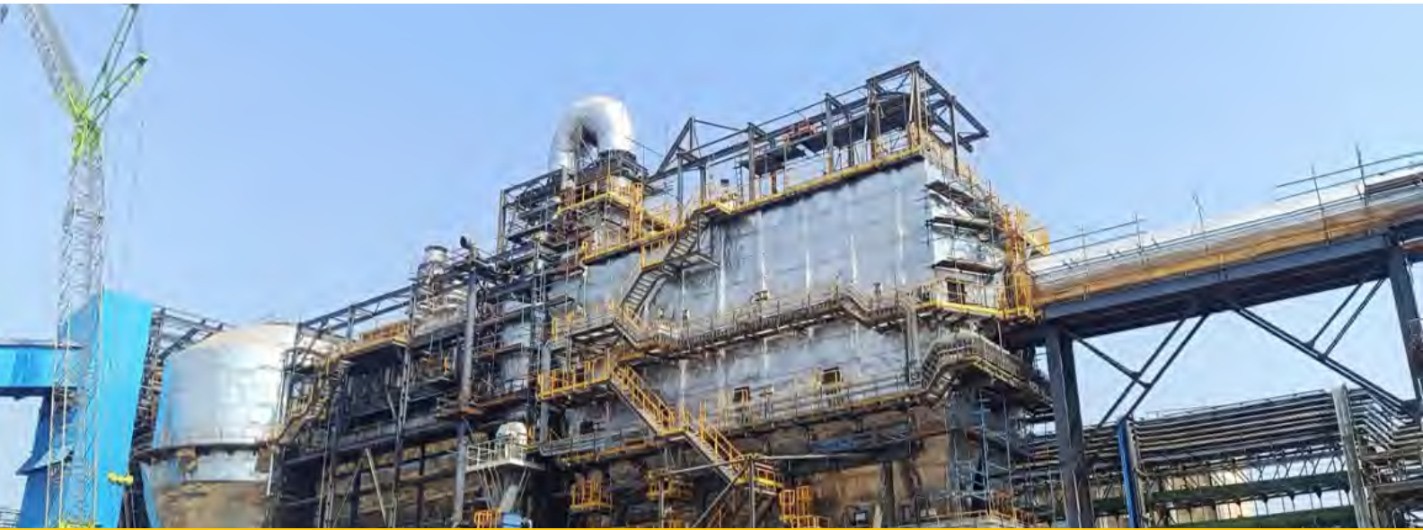
Hindustan Zinc Limited (HZL) - Upgradation of the Debari Smelter Complex, Rajasthan
