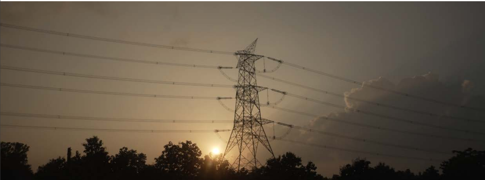
765 kV Navsari–Phadge Transmission Line, Gujarat
