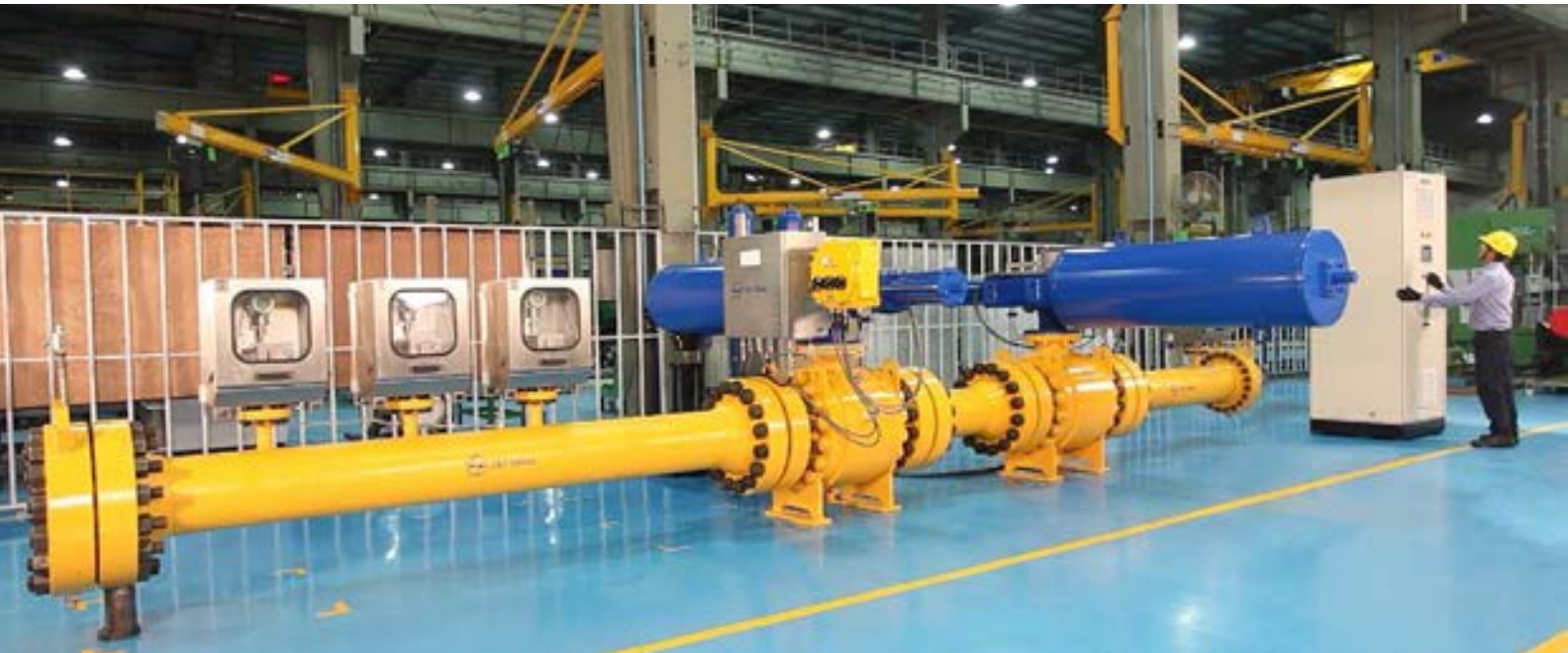
HIPPS (High Integrity Pressure Protection System) prevents catastrophic over-pressurisation and release of toxic flammable fluids
