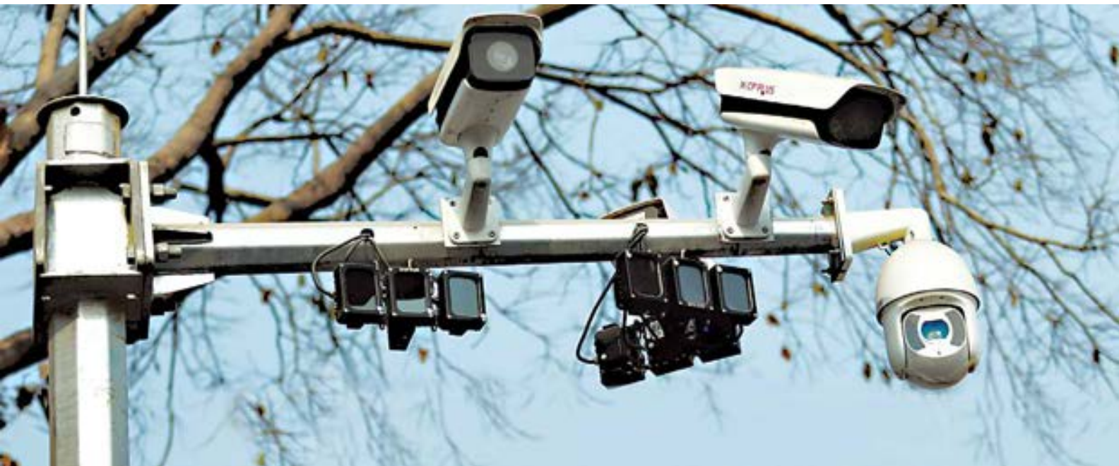
Surveillance Camera Installed at Prayagraj
