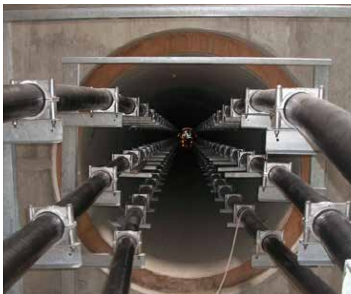
132/33 kV Underground Cable at Ghala Heights, Oman
