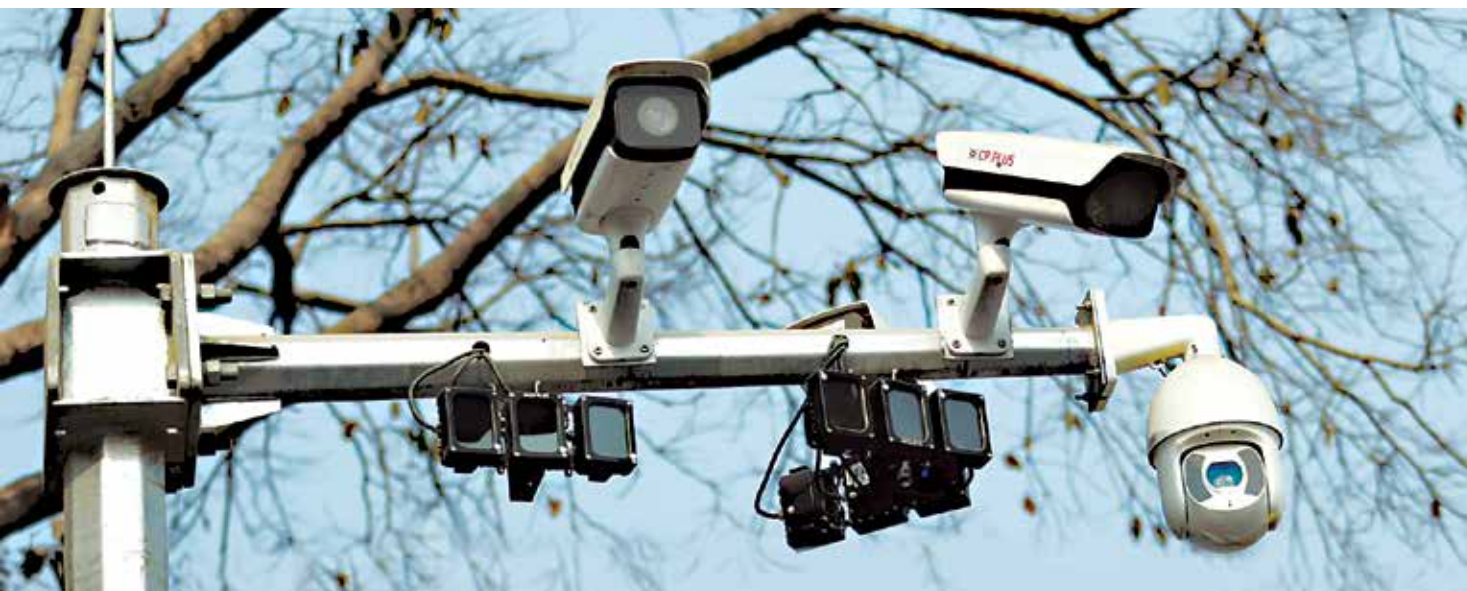
Surveillance cameras installed at Prayagraj
