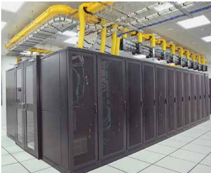
Data Center, Hyderabad
