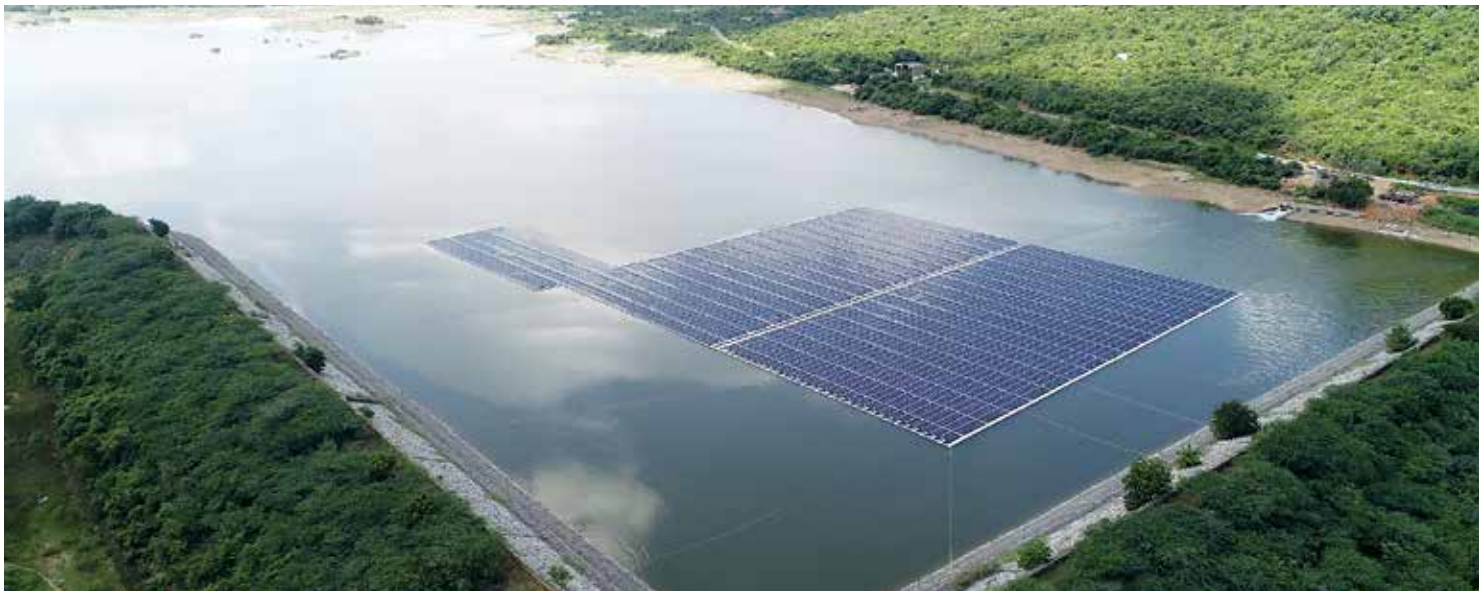
Floating Solar Project, Tirupati, Andhra Pradesh
