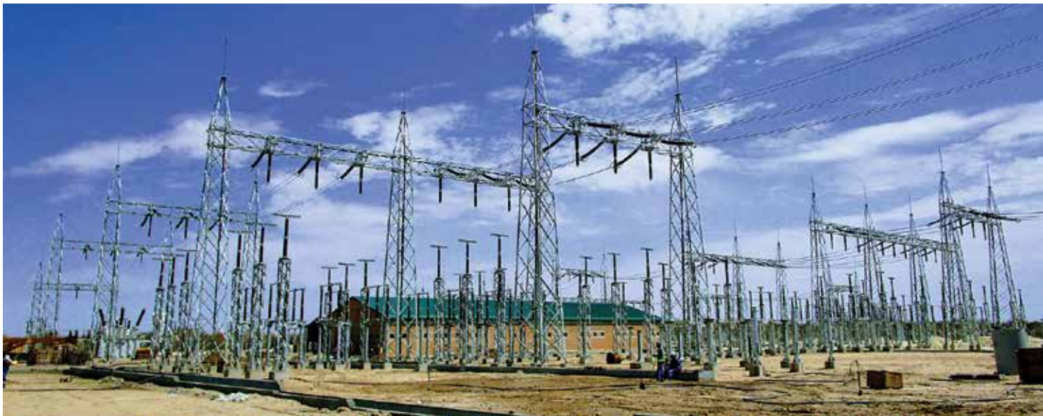
400/220/132/33 kV Substation, Mawana, Botswana
