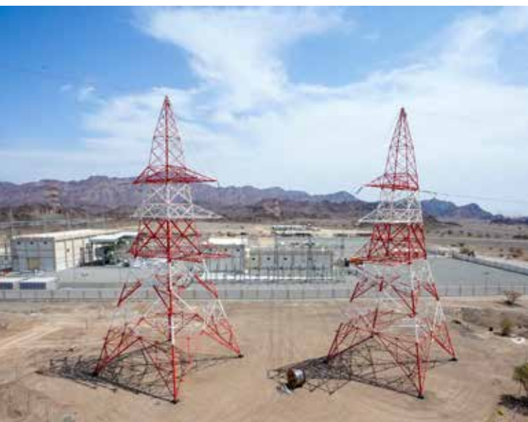
400/132 kV Grid Station at Qabel, Oman
