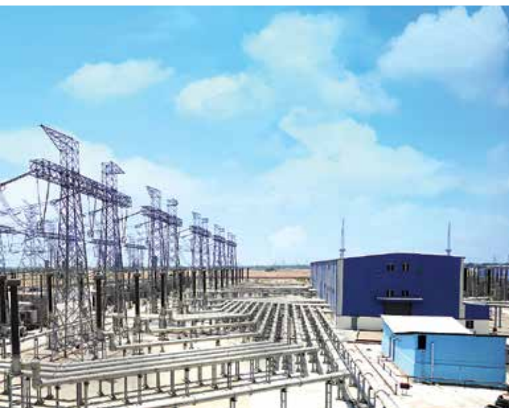
765 kV Gas Insulated Substation, Varanasi, Uttar Pradesh
