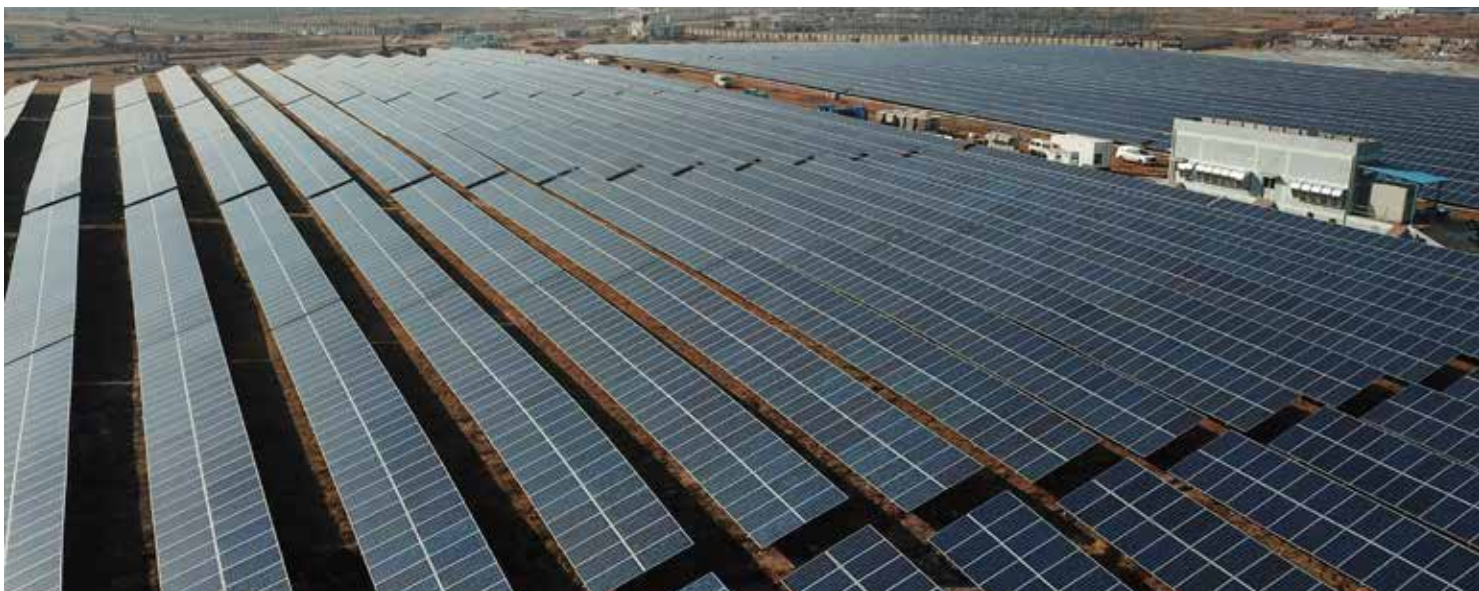
250 MWp Solar PV Plant, Madhya Pradesh
