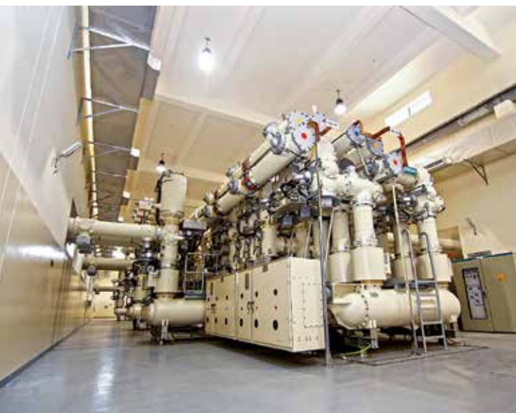
400 kV Grid Station at Misfah, Oman
