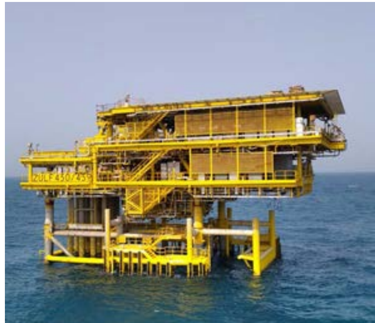
Delivered and installed two oil PDMs and associated facilities in Zuluf Fields, Saudi Arabia
