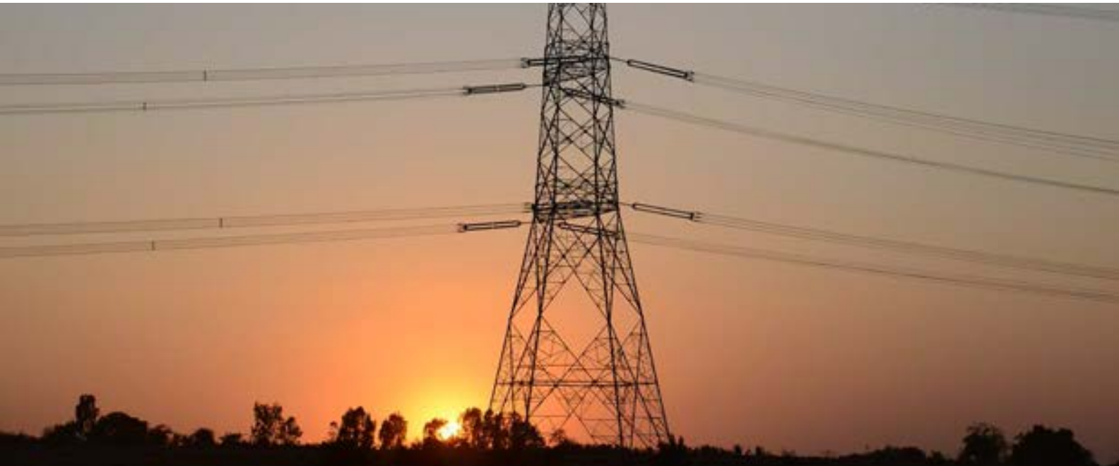
Power Transmission Tower at Kudgi Transmission Limited
