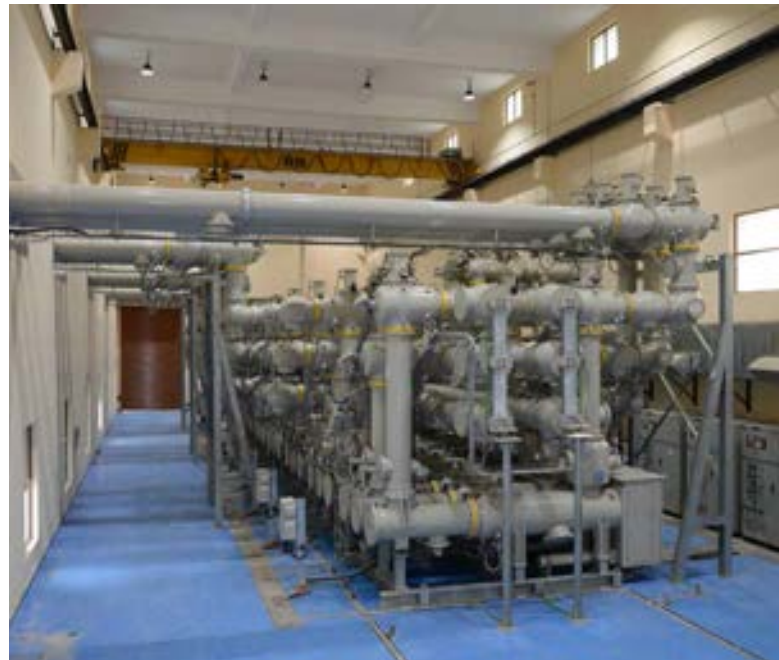
400/220 kV Mysandra GIS, Bengaluru, Karnataka
