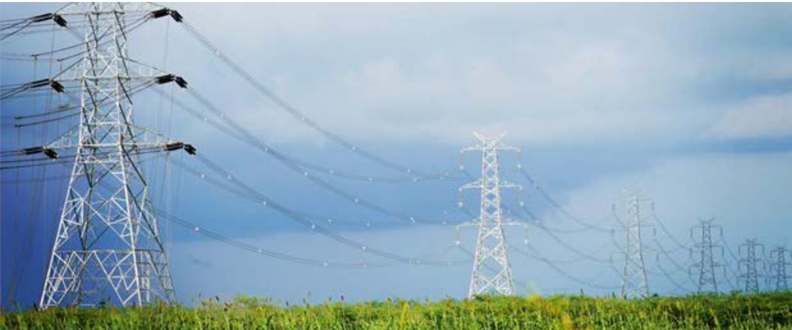
400 kV Kamudhi-Ottapidaram Transmission Line, Tamil Nadu
