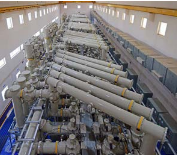
400 kV GIS Substation, Chennai, Tamil Nadu
