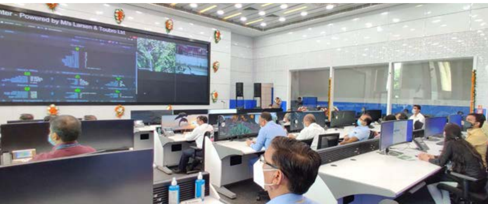
Integrated Command Control Centre for NDMC
