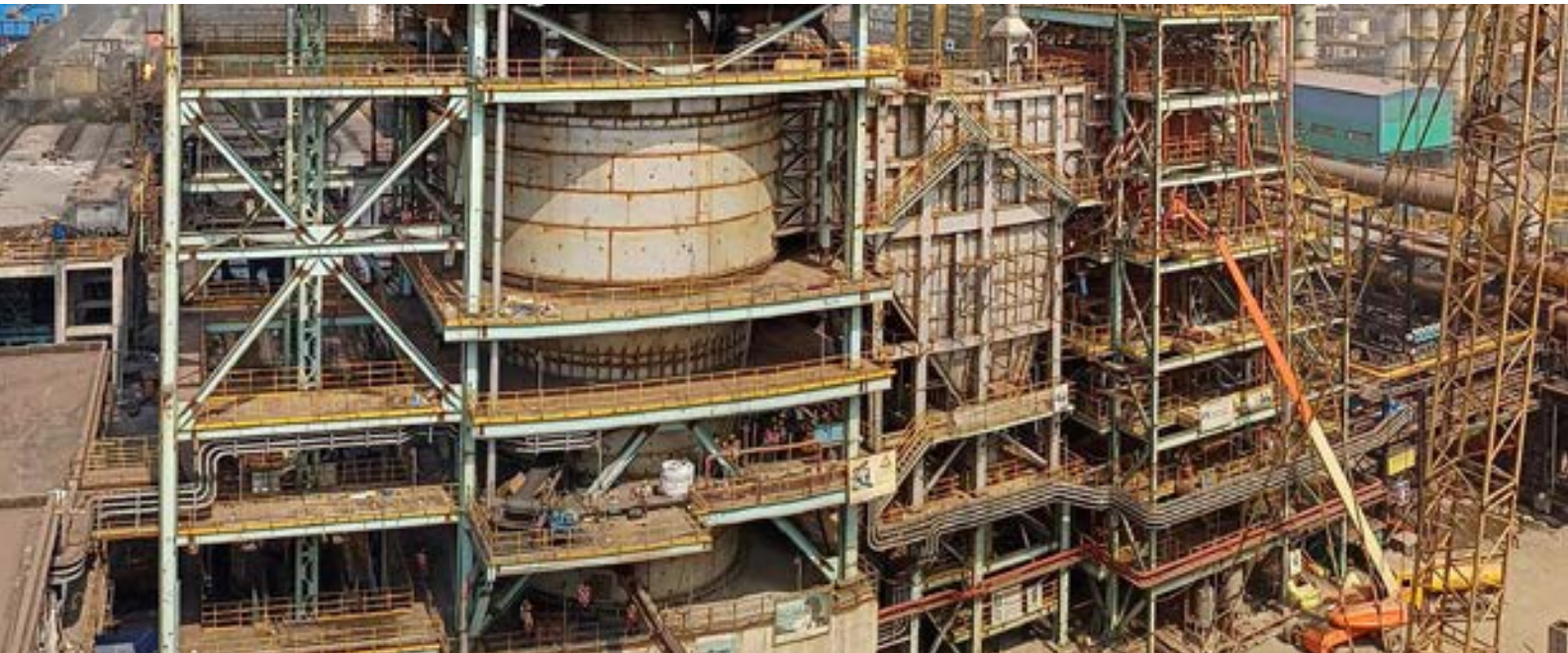
Coke dry quenching plant at JSW, Dolvi, Maharashtra
