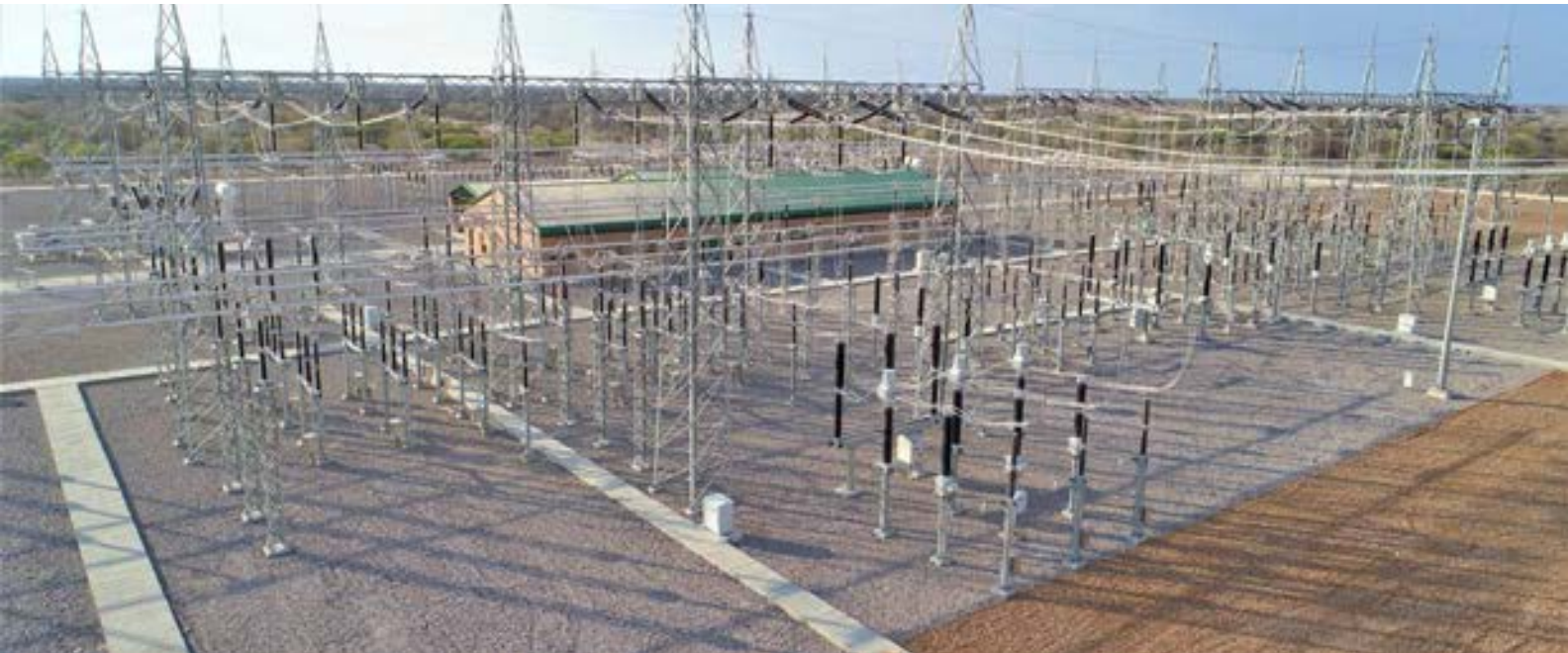
400/220/132/11 kV Mawana Substation, Botswana
