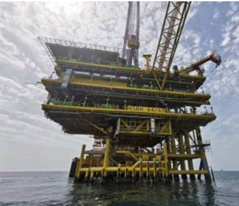
One of three gas PDMs installed in Hasbah and Arabia Offshore, Saudi Arabia
