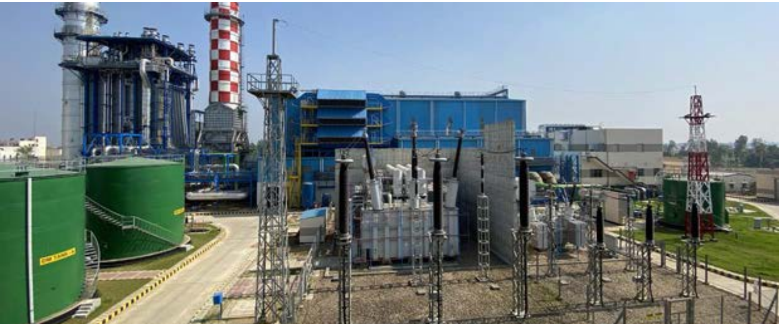
400 MW Bibiyana South Combined Cycle Power Plant, Bangladesh
