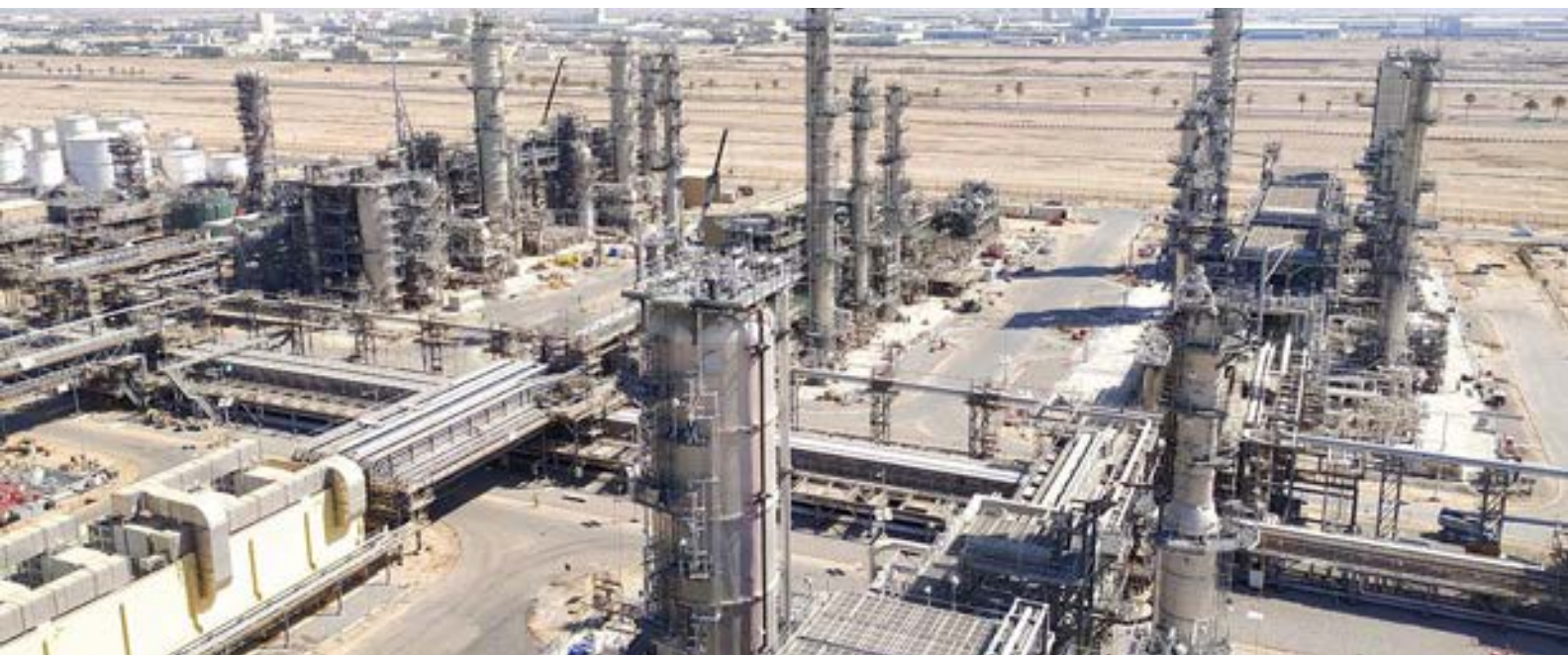
n-Paraffin & Derivative Complex for Farabi Petrochemical Company at Yanbu, KSA
