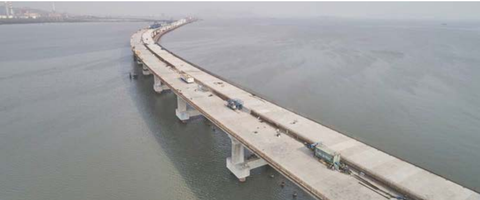
L&T is constructing 13 km of the 21-km Mumbai Trans Harbour Link – which will be India's longest sea bridge
