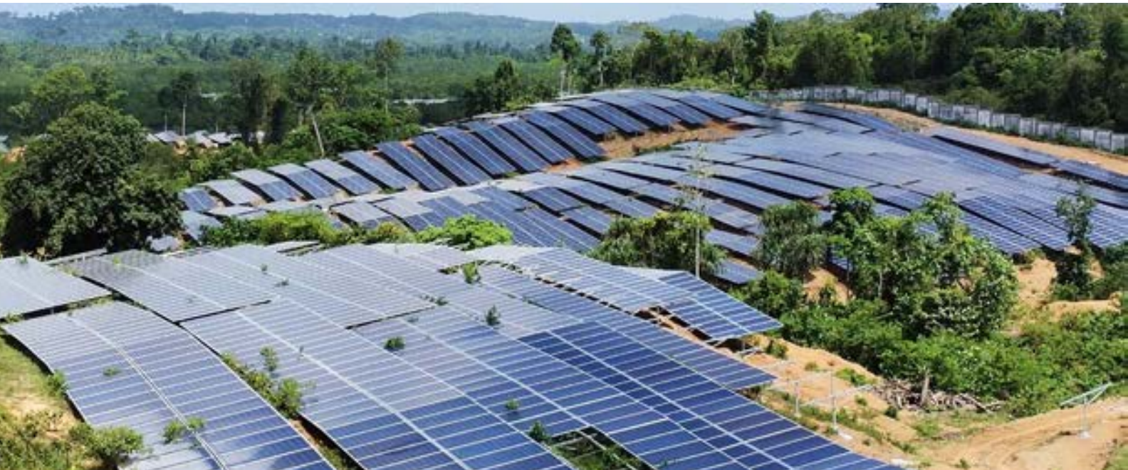
India's first large-scale solar PV project of 2 x 10 MW with 16 MW / 8 MWh battery energy storage system in the Andamans
