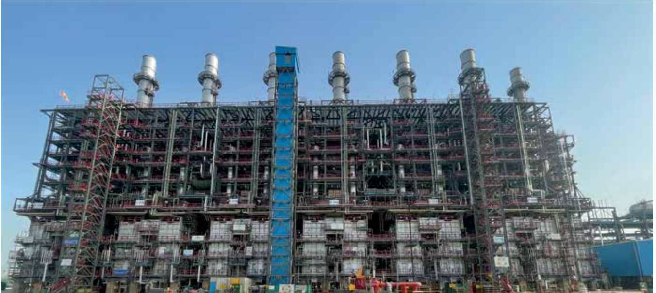
Cracker Furnace Package for HPCL-Mittal Energy Limited (HMEL) at Bathinda
