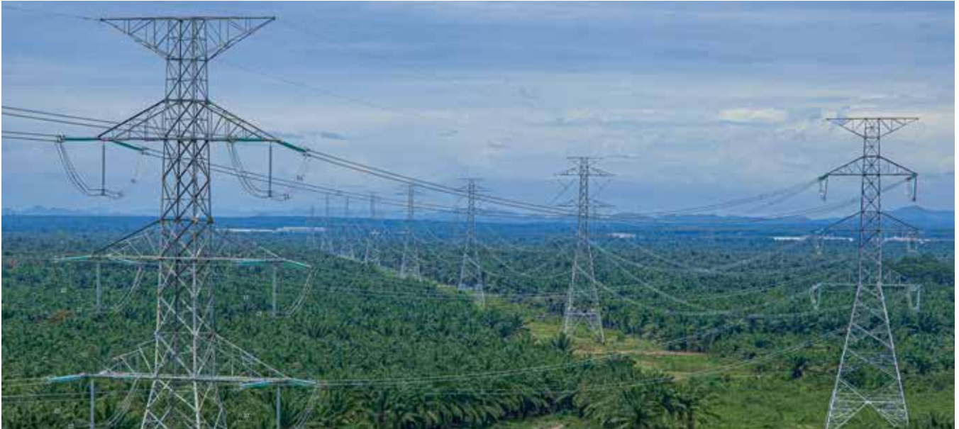
500kV Bang Saphan 2 to Surat Thani 2 Transmission Line
