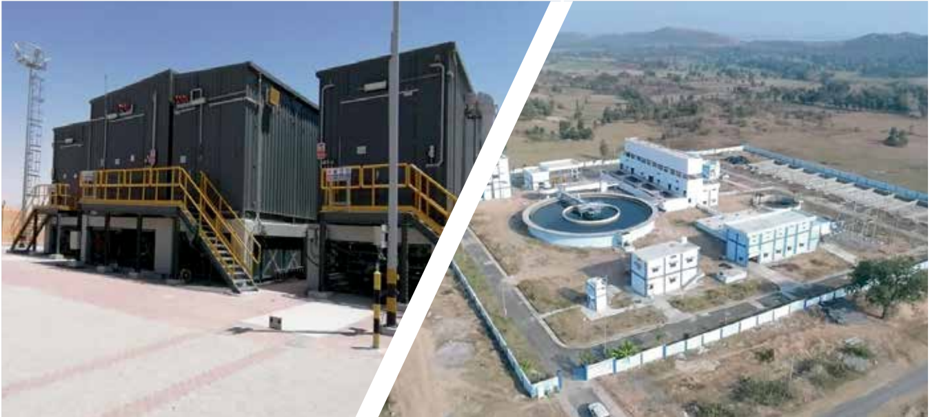
Haliba, Containerised Substation
