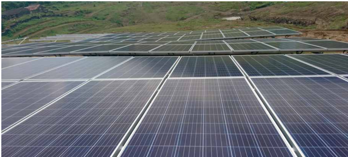
Large scale solar cum storage project in Andaman
