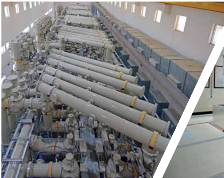
400 kV GIS Substation, Chennai, Tamil Nadu
