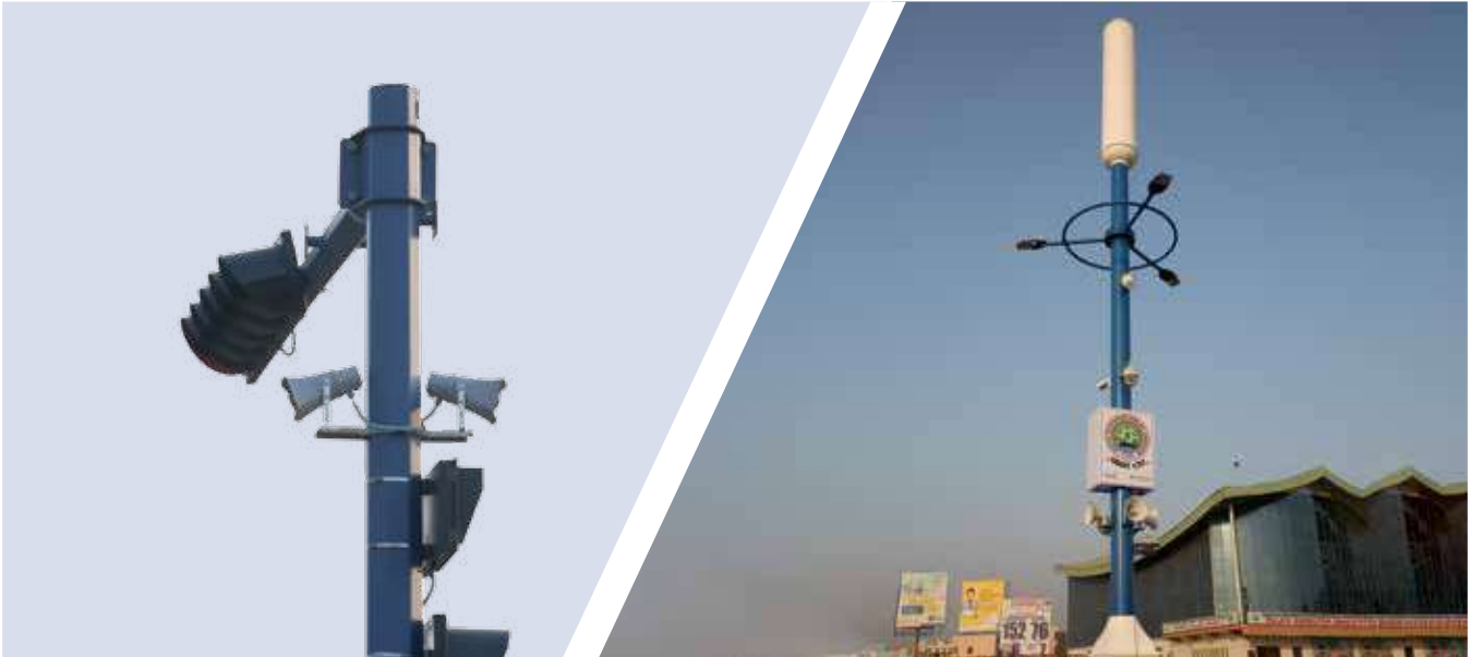
Smart Signalling System at Raipur
