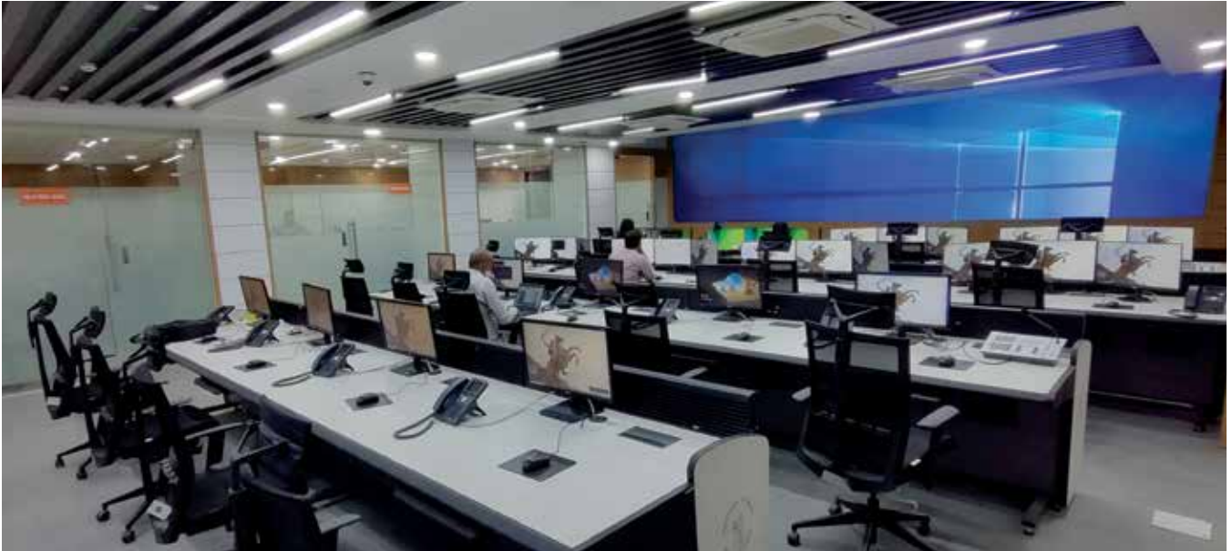
Integrated Command Control Centre, Jhansi
