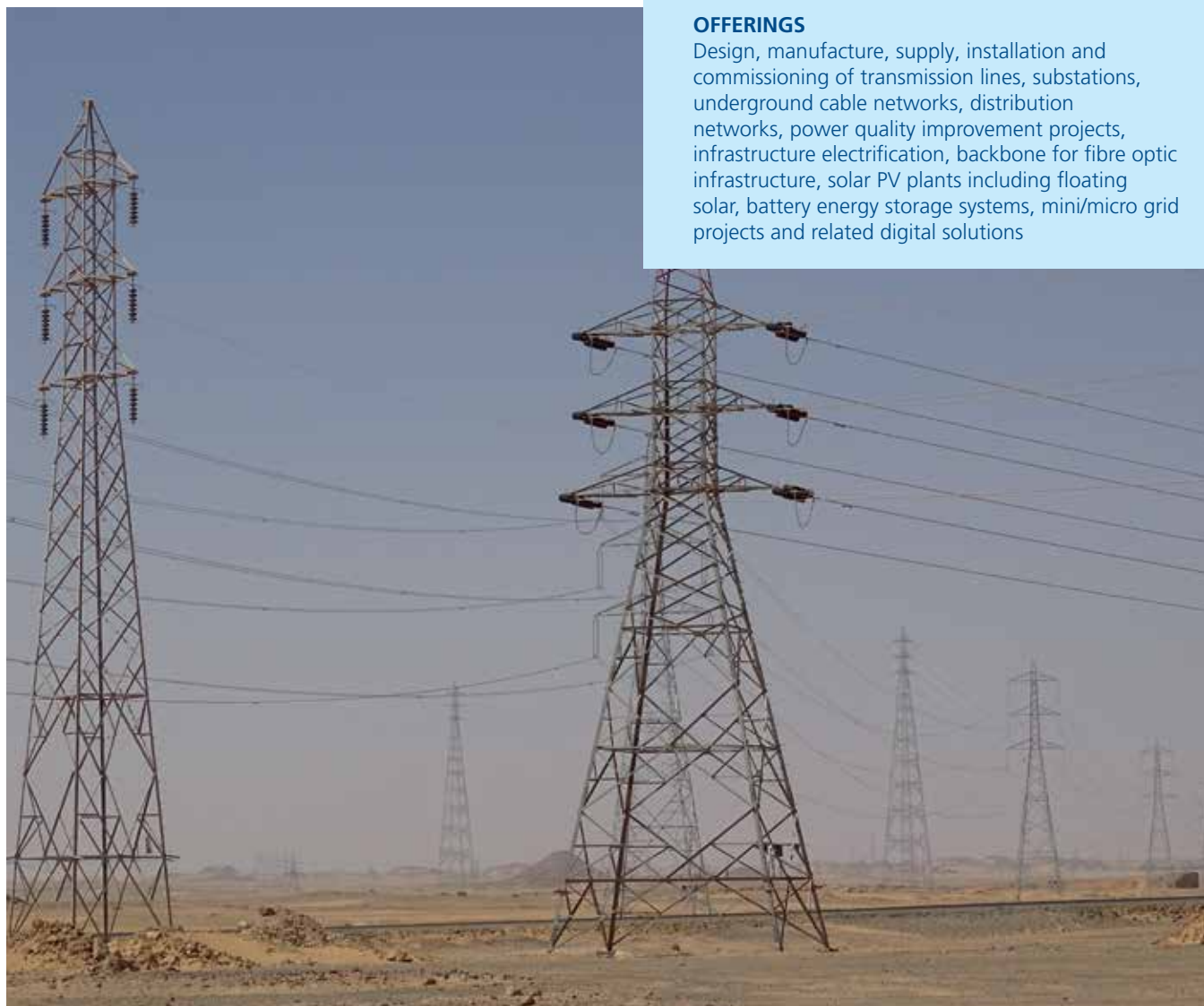
Toshka 2 – Wadi Halfa 220 kV double circuit overhead transmission line, Egypt
