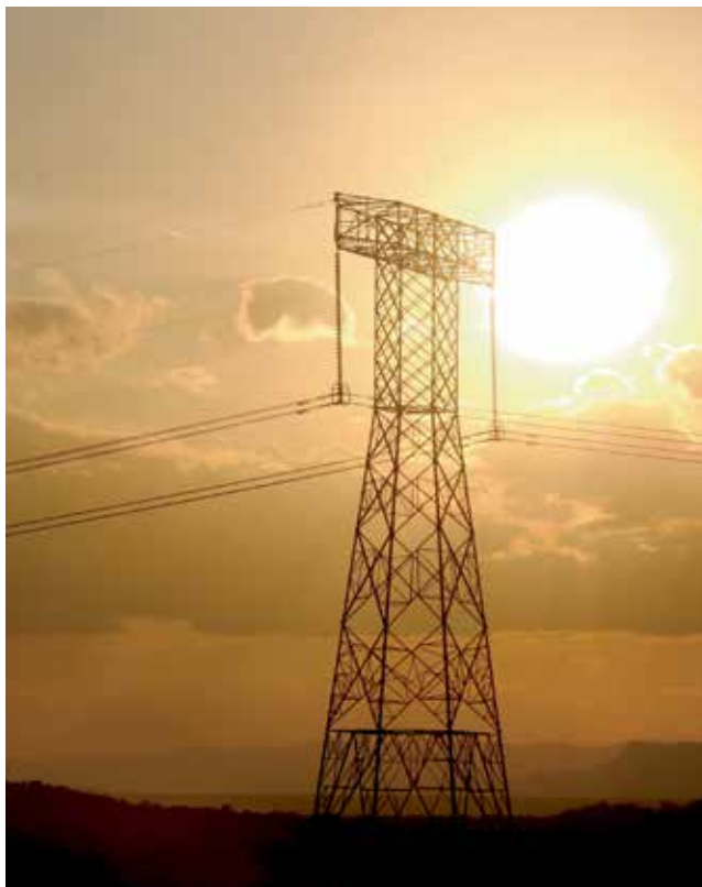
400 kV Ibri Izki Transmission Line, Oman
