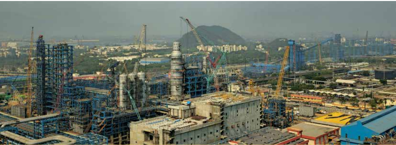
Residue Upgradation Facility (RUF) for HPCL, Vizag, Andhra Pradesh
